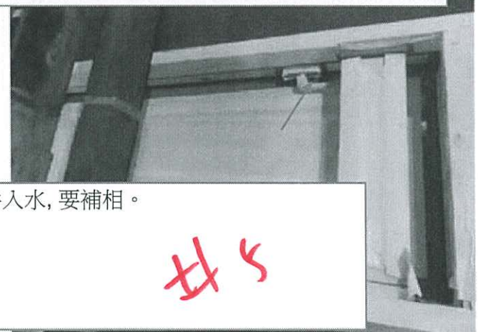
26_15F-T1BCW4 AS-01 water leakage
