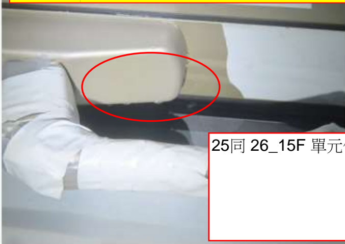
25_15F-T1BCW4 AS-01 water leakage
