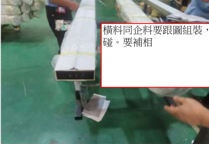
3_ one side of mullion was found consealed
