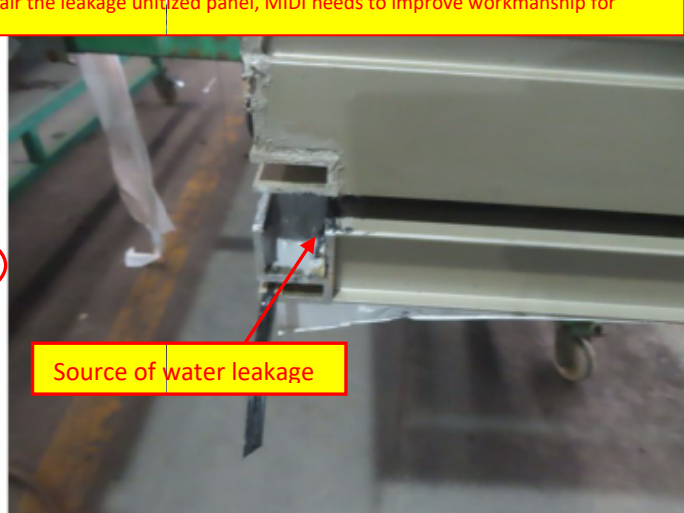
20_Damage sealant was found at end position of mullion
