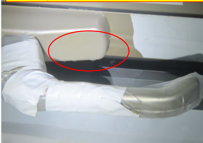
25_15F-T1BCW4 AS-01 water leakage
