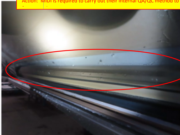
19_Water leakage was found inside spandrew backpan
