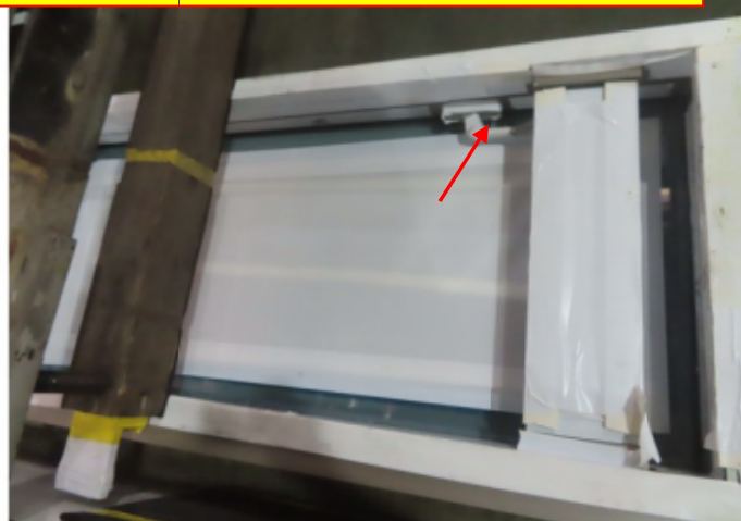
26_15F-T1BCW4 AS-01 water leakage
