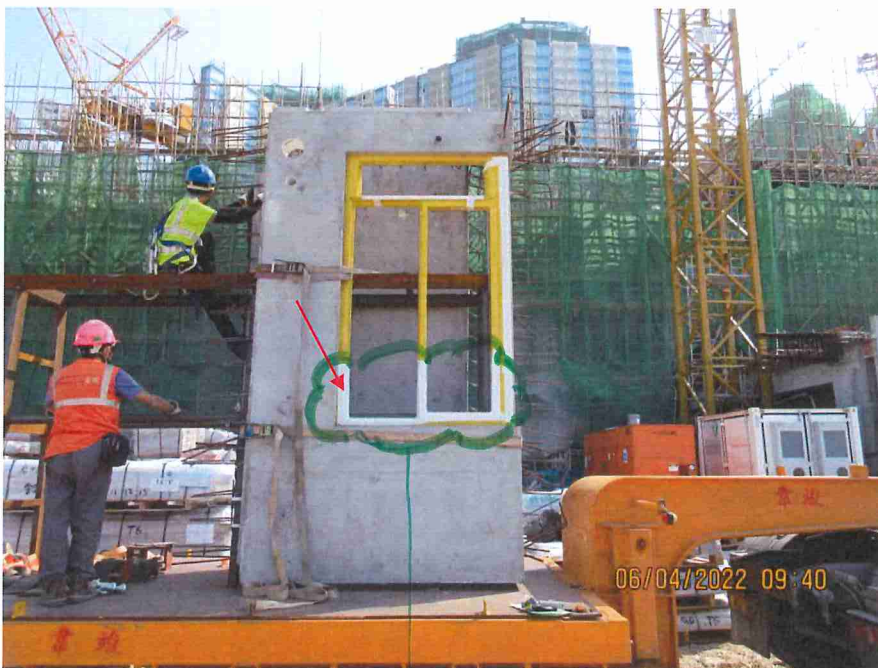
Plastic cover was provided on lower part of aluminum window frame
