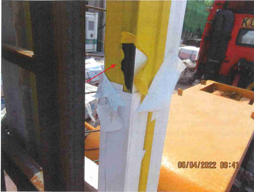
Only provide one layer plastic sheet to upper part of aluminum window frame
